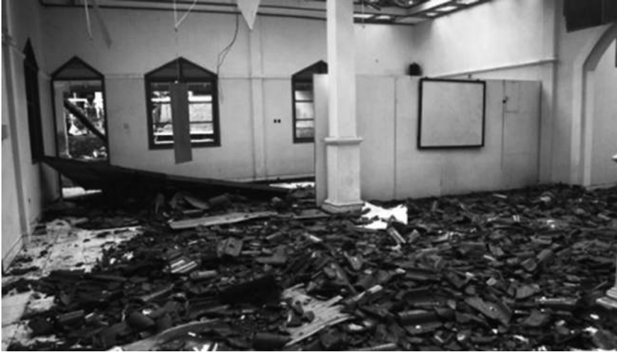
The condition of Nurhidayah Mosque belong to Ahmadiyah followers after destruction in Cisaar, Cipeuyeu, Cianjur, West Java, on Saturday, February 8th, 2012. (Picture: TEMPO/Prima Mulla).
